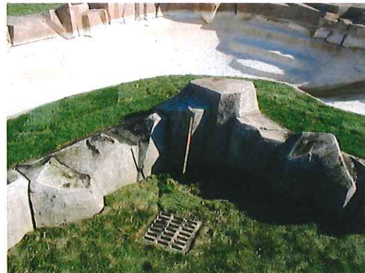
Area drain with installed turf
