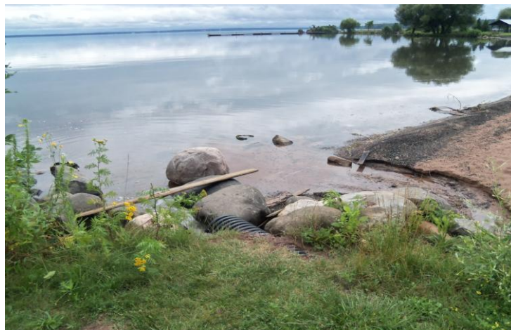
Photo 56: Stormwater outfall (Pipe 1) at the east end of the beach (potential pollution source).
